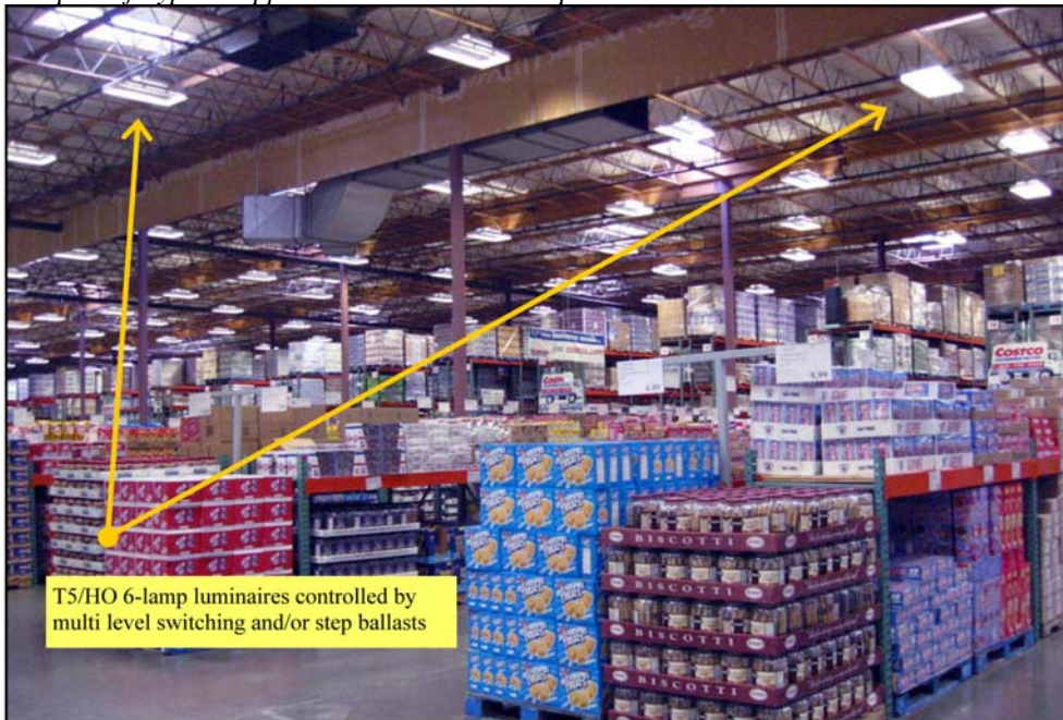
BIG BOX RETAIL ( minimal or no daylight harvesting ) can Load Shed 20% to 25% through use of comprehensive lighting controls coupled with Demand Response controls. Night time adaptive illumination ( also possible with this system ) could result in a 33% low LPD during evening hours. Night time adaptive reduction as well as most load shed scenarios are achieved while maintaining IES-RP2 minimum illumination targets.
