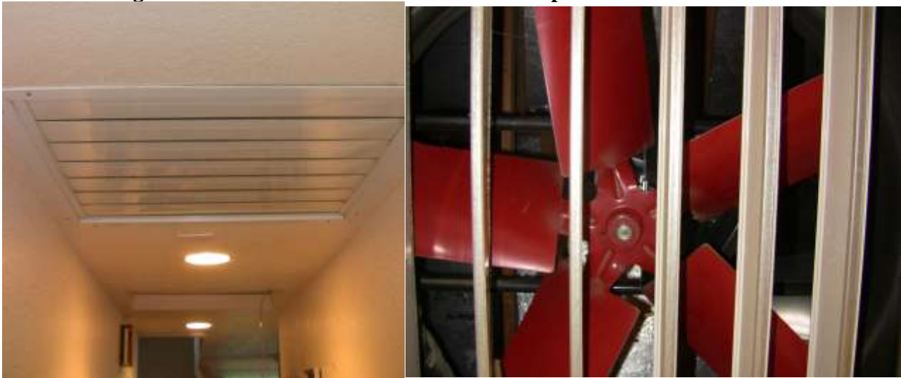
Figure 1: Whole House Fan Barometric Damper and Motor/Fan in Attic
