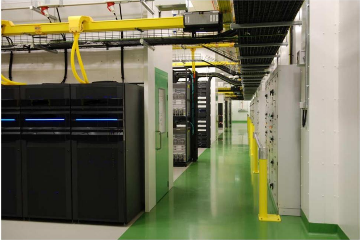
Figure 20. Example Containment System – Custom Hot Aisle Enclosures
