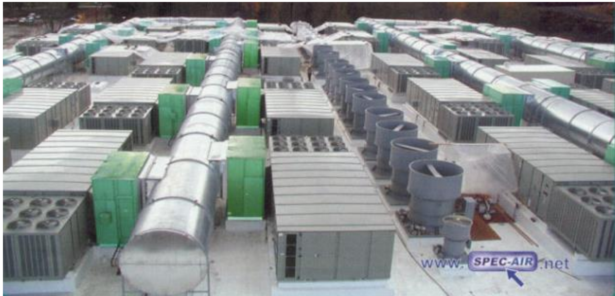
Figure 18. Data Center with Direct Evaporative Humidification
