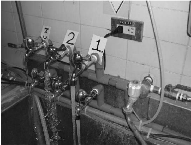
FIGURE. Experimental set up of the model plumbing system (1, faucets with aerators; 2, control faucets; 3, faucets with laminar water flow devices).
