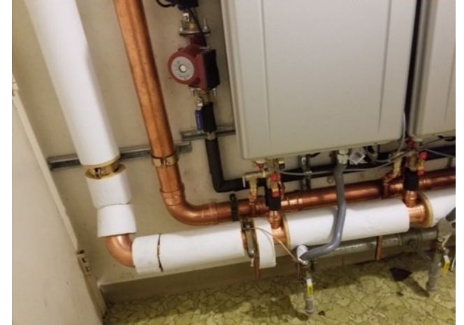
Uninsulated Fittings and Valves
