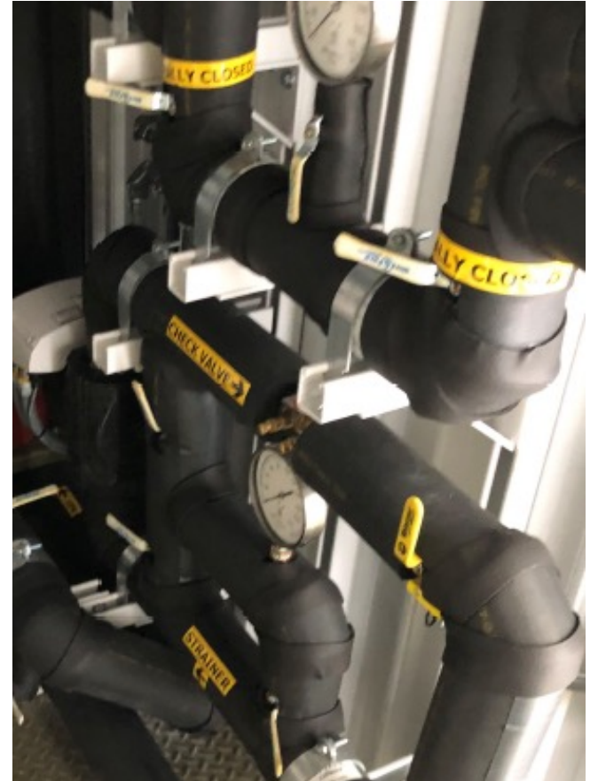
Uniform Pipe Insulation Across Piping, Valves and Fittings
