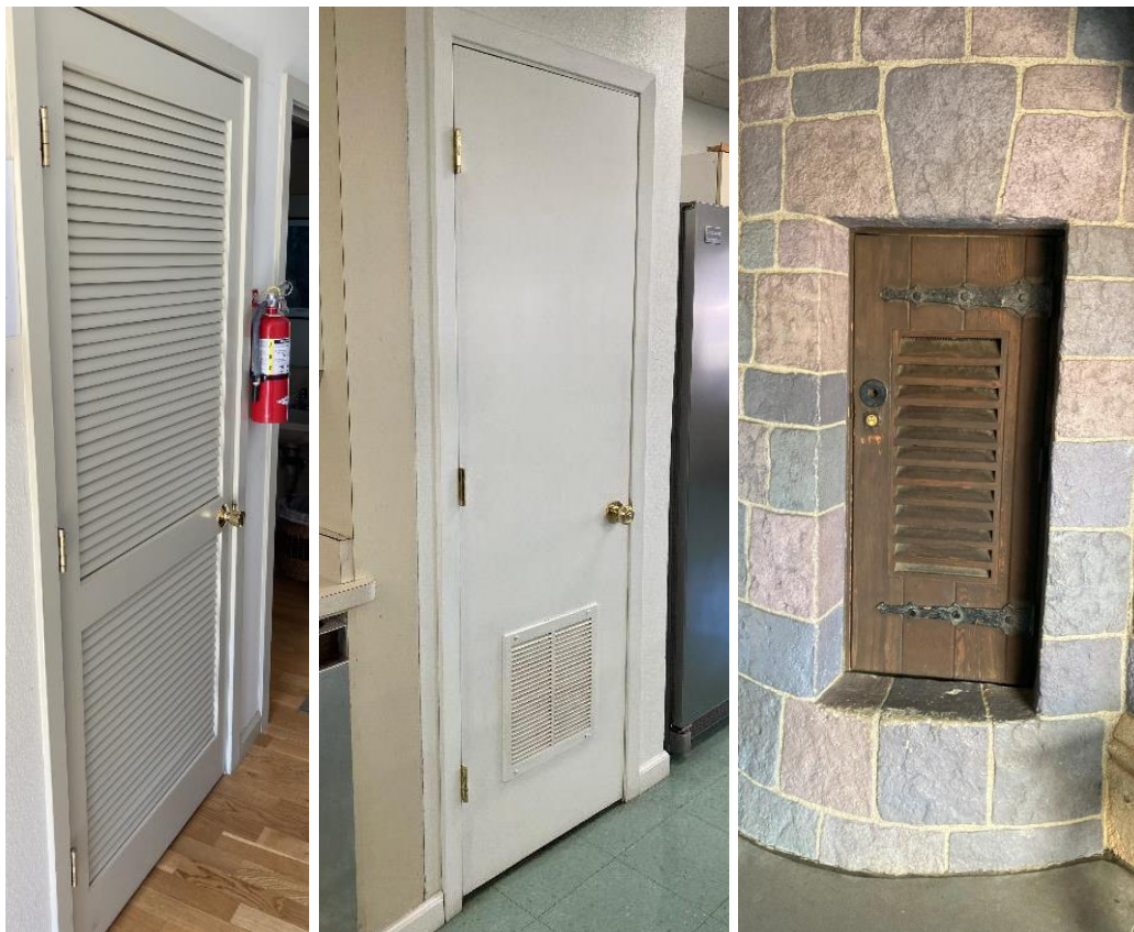
Figure 44: Left, 34-year-old fully louvered door from a small office in Davis, CA. Middle, over 40-year-old DHW closet door with retrofit lower grilles from a small commercial kitchen in Woodland, CA. Right, over 60-year-old wood door with louvered section in Anaheim, CA.
