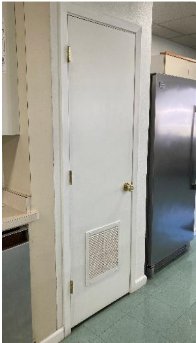
Figure 22: DHW closet door with lower grilles from a small commercial kitchen in Woodland, CA.
