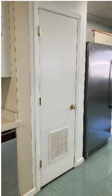
Figure 22: DHW closet door with lower grilles from a small commercial kitchen in Woodland, CA.
